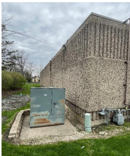
Water damage from drainage issues
