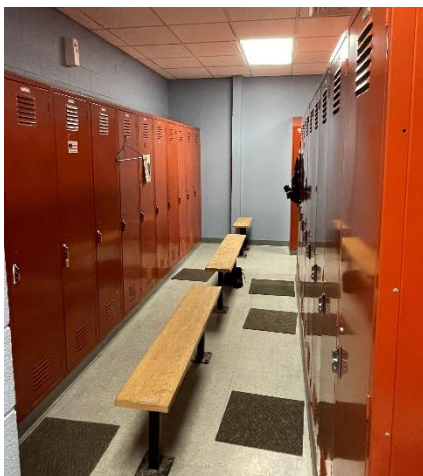
Inaccessible lockers and benches in locker room
