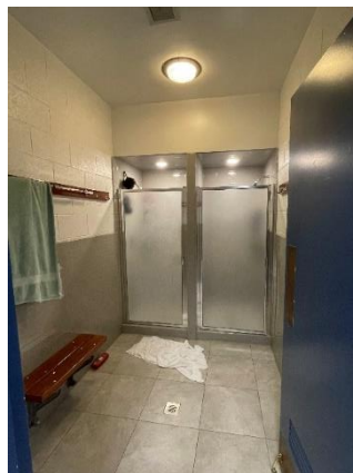
Non-ADA compliant showers within men’s locker rooms
