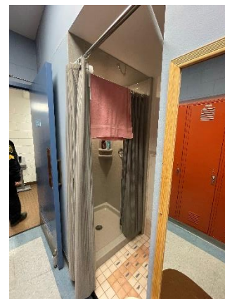
Non-ADA compliant showers within women’s locker rooms
