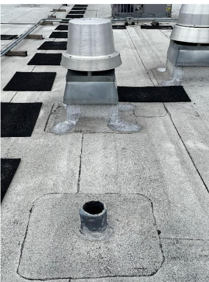
Deteriorated flashing at roof curbs
