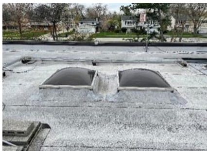
Deteriorated flashing at skylights
