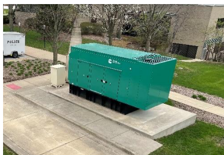
Village Hall generator
