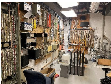
Older fire alarm and phone wiring
