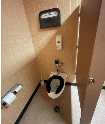
Non-ADA compliant toilet room
