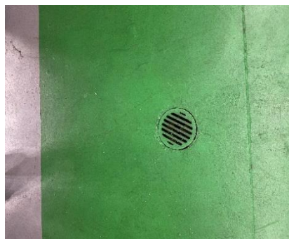
Floor drain in Firing Range
