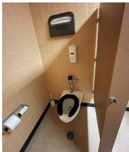
Non-ADA compliant toilet room
