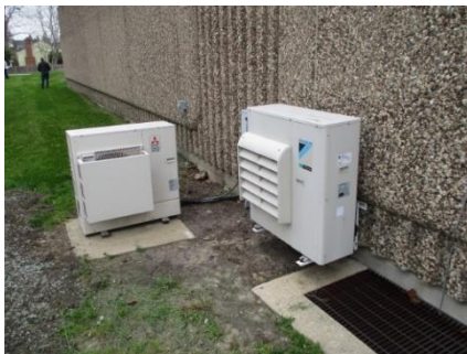
Ductless split units
