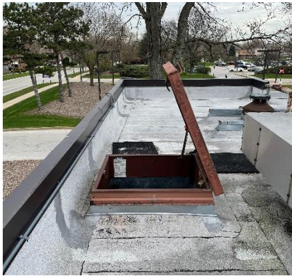
Roof hatch too close to roof edge.
