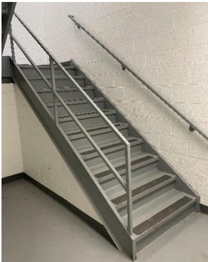
Non-ADA compliant guardrail
