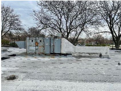
Existing air handler
