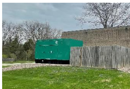
Police Department generator
