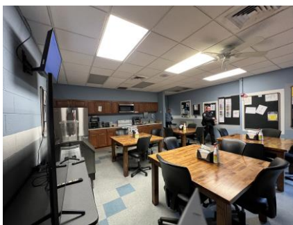
Older fluorescent lighting fixtures
