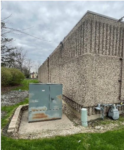
Transformer & retaining wall
