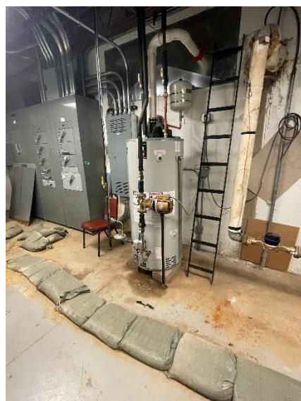
Main electrical service
