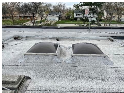
Deteriorated flashing at skylights
