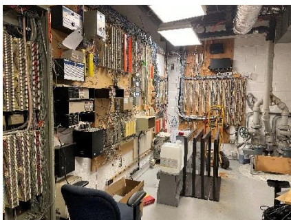
Fire alarm and phone system
