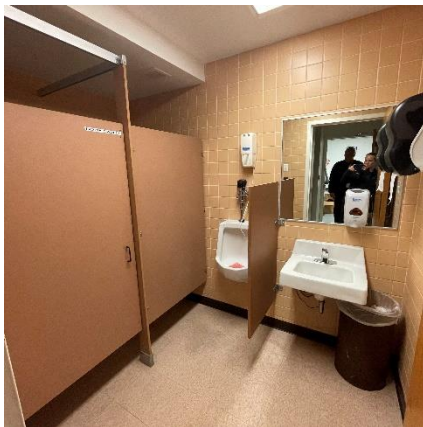
Non-ADA compliant toilet room
