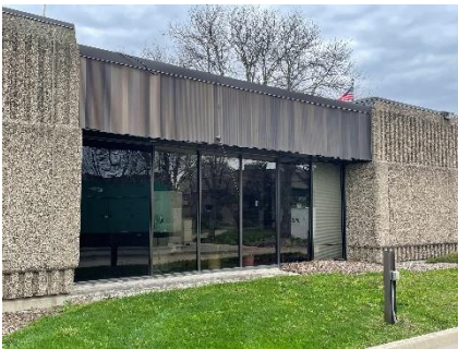
Damaged siding at west side
