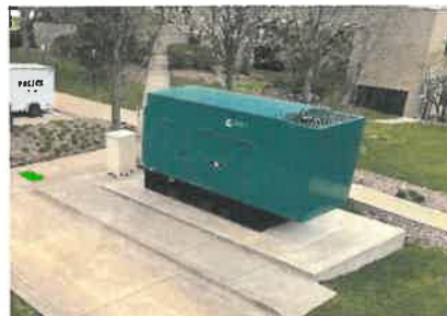
Village Hall generator
