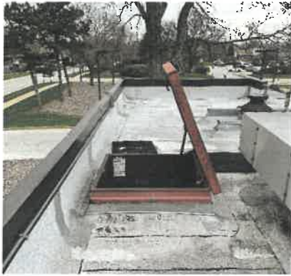
Roof hatch too close to roof edge.
