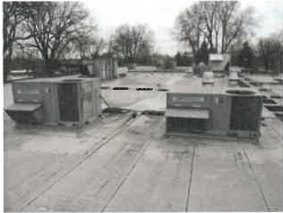
Existing rooftop units
