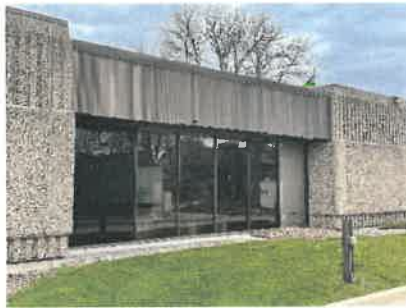
Damaged siding at west side
