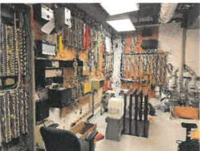
Fire alarm and phone system
