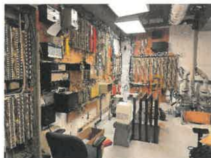
Older fire alarm and phone wiring
