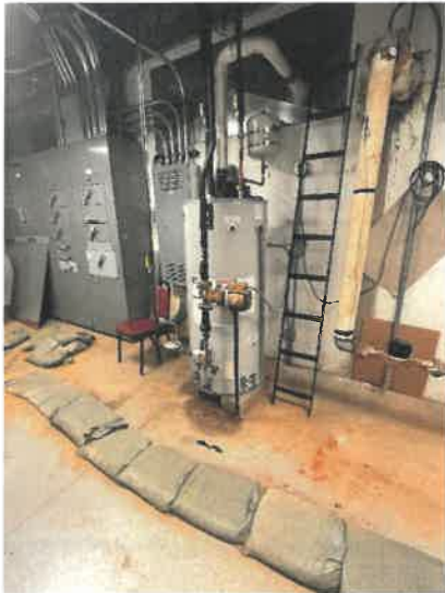
Electrical service with sandbags to keep water away
