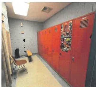
Inaccessible lockers and benches in locker room
