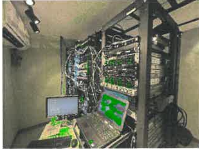
IT Racks in server room
