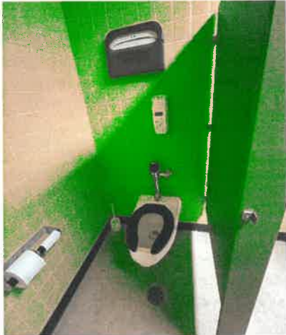
Non-ADA compliant toilet room
