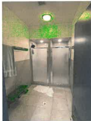
Non-ADA compliant showers within men's locker rooms
