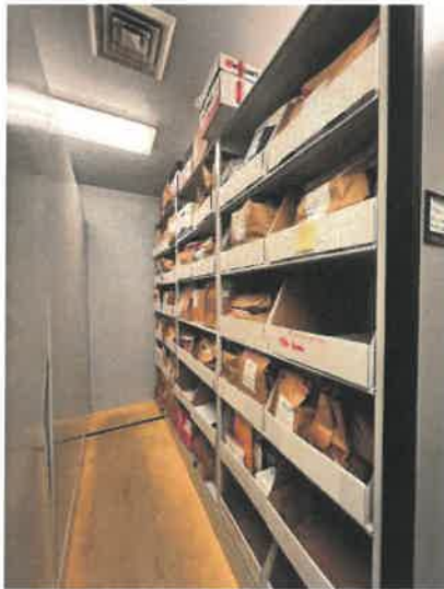
Insufficient ventilation in Evidence Storage room
