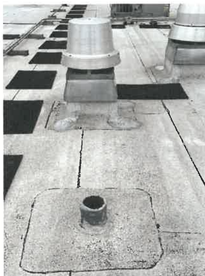
Deteriorated flashing at roof curbs
