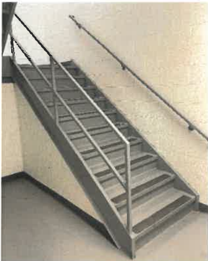
Non-ADA compliant guardrail
