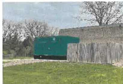
Police Department generator
