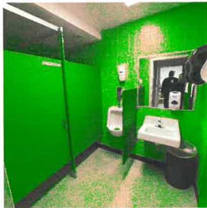
Non-ADA compliant toilet room
