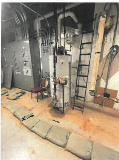
Main electrical service
