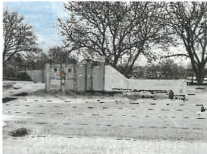
Existing air handler
