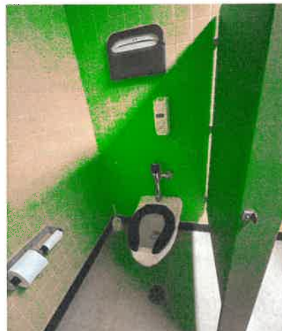
Non-ADA compliant toilet room
