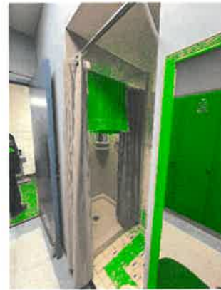
Non-ADA compliant showers within women's locker rooms
