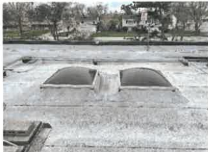
Deteriorated flashing at skylights
