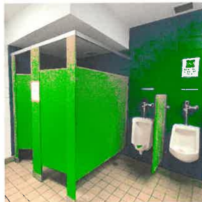
Non-ADA compliant toilets within men's locker room
