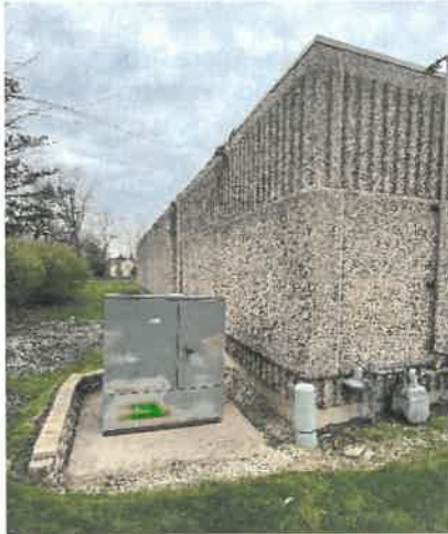
Transformer & retaining wall
