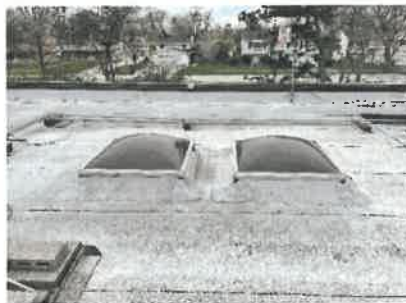
Deteriorated flashing at skylights
