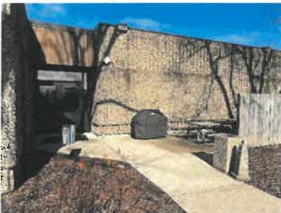
Existing exterior light fixtures
