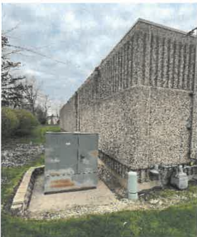
Water damage from drainage issues
